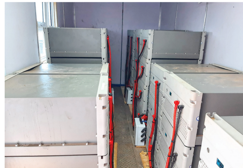
Solar mini-grid battery bank in Buna, Wajir County.
