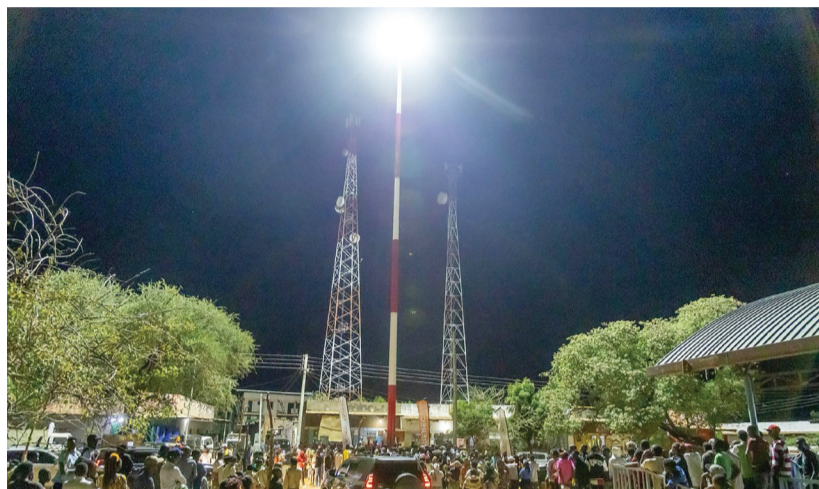
High mast flood lights in Embakasi South Constituency, Nairobi County.
