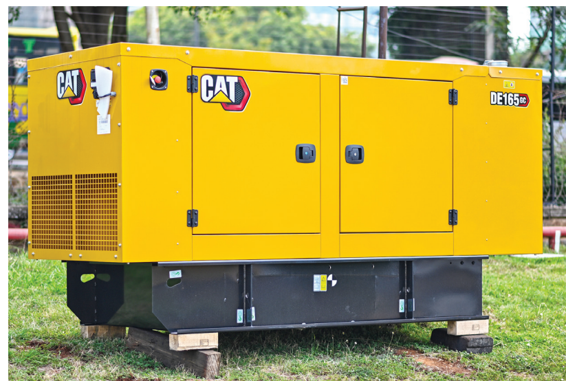
Caterpillar Canopied generator. PHOTO | MANTRAC KENYA
